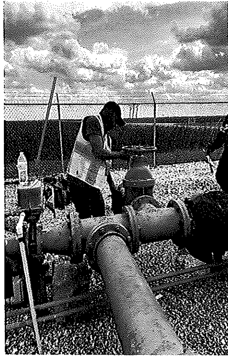
Figure 1: MOV 2 Near to Small Storage Tank
